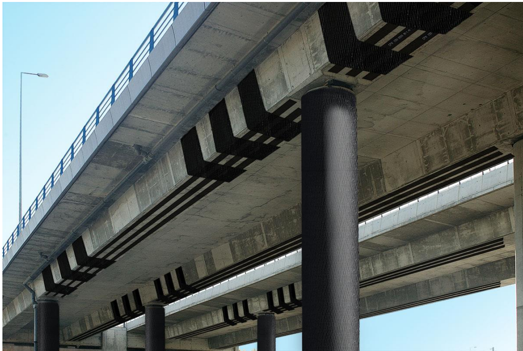
Figure 5.16: Carbon Fiber Reinforced Polymer (CRP) stripes for the reinforcement of a bridge.
