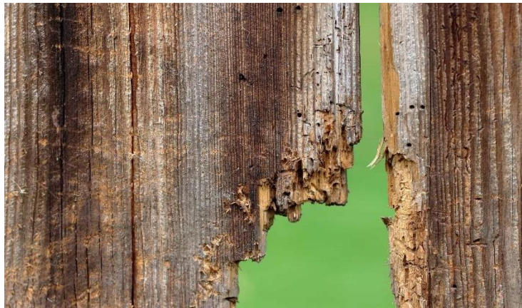
Figure 1.9: Wood damaged by mold
